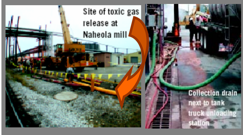
This accident investigated by and pictures provided by the U.S. Chemical Safety and Hazard Investigation Board. Visit their site at http://www.csb.gov
